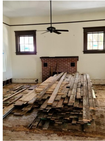
Floors of Historic Palm Cottage post Hurricane Ian
