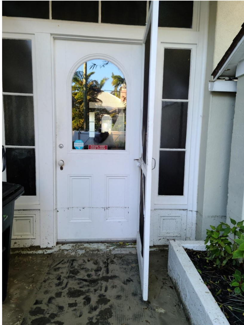
Back door of the Cottage...notice the water/mud surge line.
