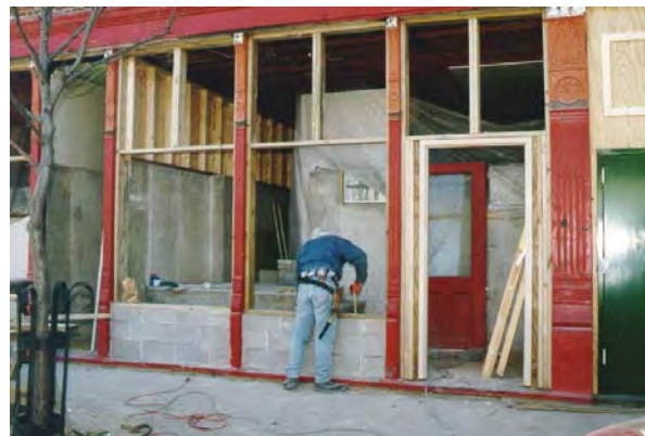
Floodproofing the vestibule of a storefront
